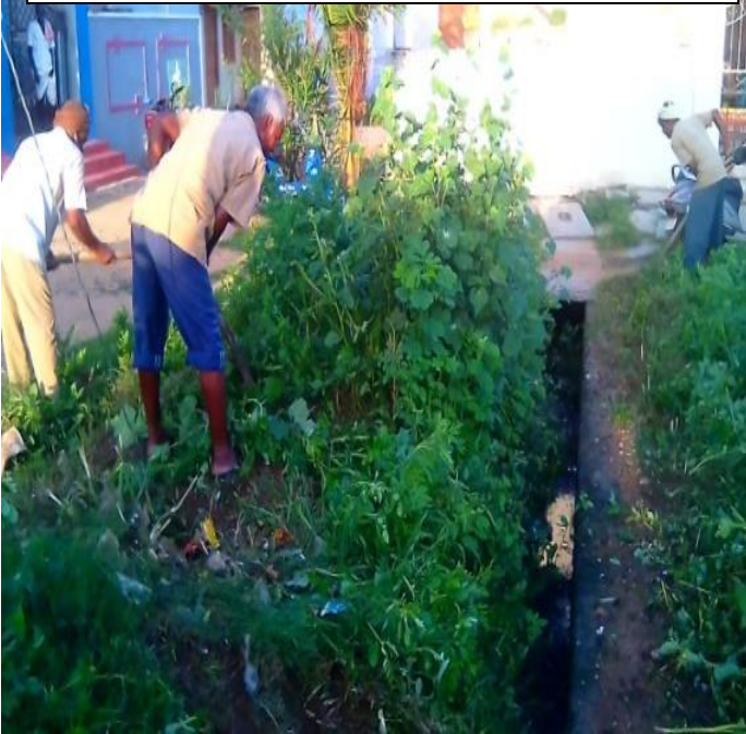
BEFORE W.NO.21, ESHWAR MANDIR BACK SIDE
